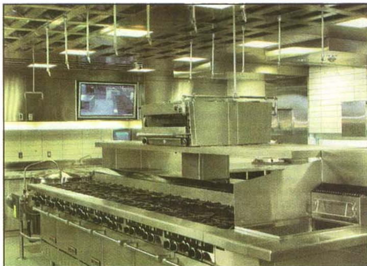
No hoods: The Vent Master ventilated ceiling at Humber College, a cooking school based in Toronto, Canada. Air is pulled through small openings in the ceiling, and vapors are trapped in dishwasher-safe cartridges. The hanging rods are a fire safety feature. The first U.S. model is being installed at the new Westin Hotel in Minneapolis, set to open in March.
